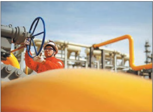
An employee checks a gas storage facility in Binzhou, Shandong province. DU PENGHUI / XINHUA
