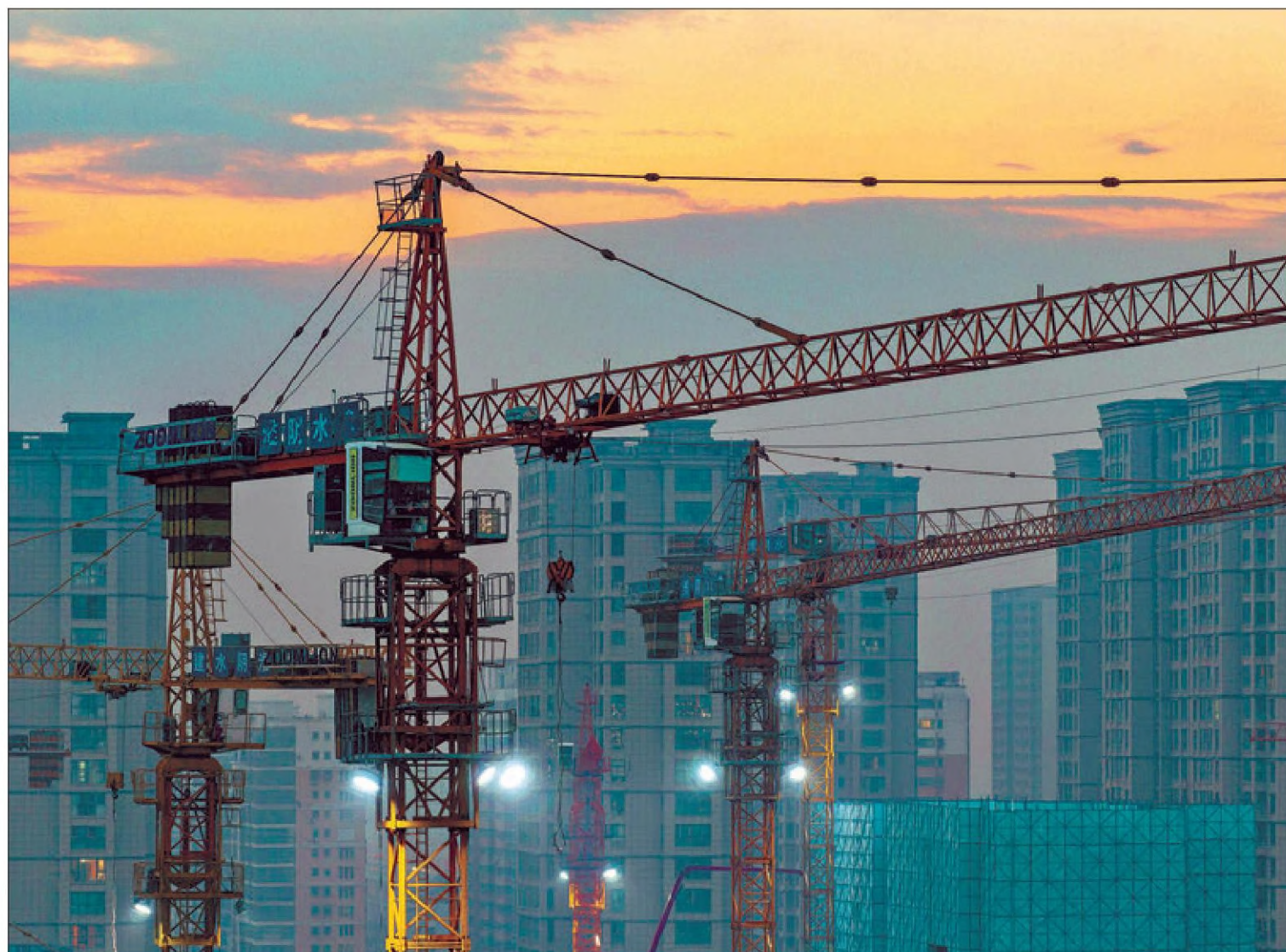
A view of a real estate construction site in Huai'an, Jiangsu province, in December. PROVIDED TO CHINA DAILY
