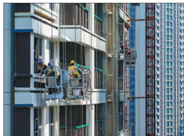
Workers are seen busy at a construction site in Huai'an, Jiangsu province, in December. PROVIDED TO CHINA DAILY
