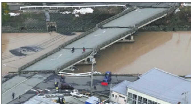
Left: Cracks are seen on a bridge following an earthquake in Suzu, Ishikawa prefecture, Japan, on Tuesday. KYODO NEWS VIA AP
