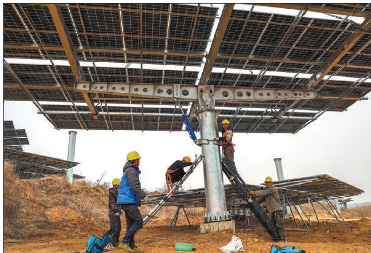
Workers install photovoltaic panels at a farm in Qingdao's West Coast New Area, Shandong province, in March 2022.
