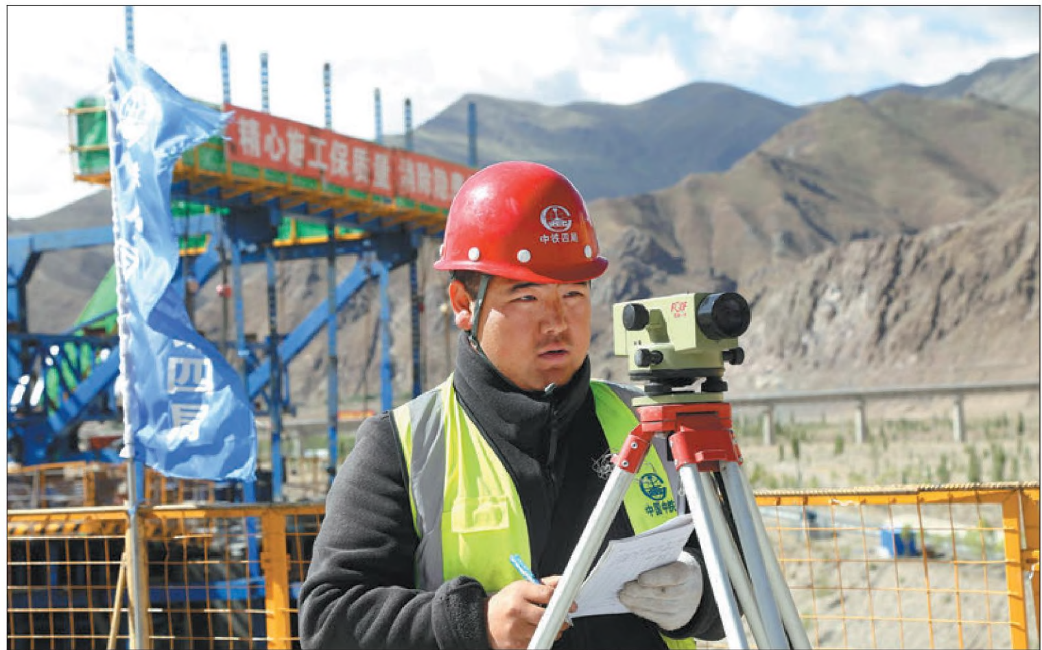
Tenzin Phuntsog, a native of Sog county, Xizang autonomous region, and an employee of China Railway No 4 Engineering Group Co Ltd, takes measurements at the construction site of the Lhasa-Shigatse Expressway. PROVIDED TO CHINA DAILY
