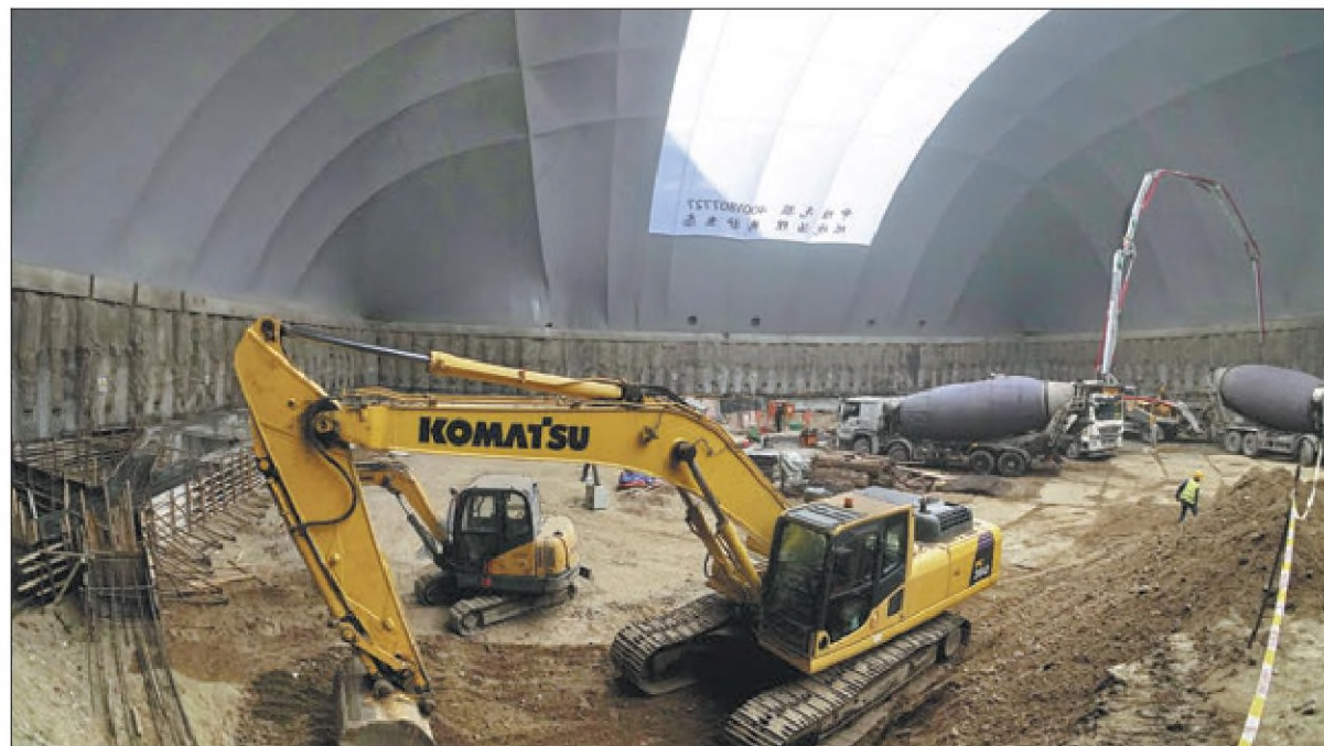
A giant air-supported membrane structure covering an area of 4,240 square meters is erected at a construction site in Beijing to prevent dust raised during construction work from polluting the air. LI XIN / XINHUA
