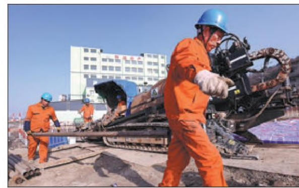
Employees of State Grid Zhoushan Power Supply Co ready cable for an inter-island power transmission network in Zhoushan, Zhejiang province, last week. YAO FENG / FOR CHINA DAILY
