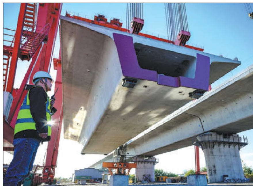
A technician guides the installation of a bridge beam at the construction site of the Hefei-Xinyi High-speed Railway in Anhui province in November. LIU YUCAI / XINHUA
