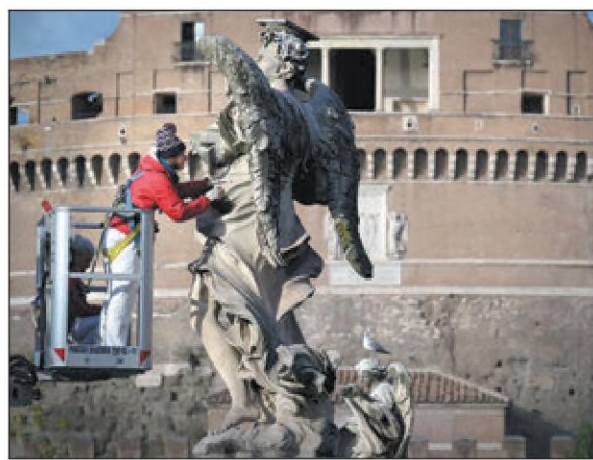
An expert restores one of the 12 angel statues on the Ponte Sant'Angelo bridge in Rome, Italy, on Monday. The Roman pedestrian bridge was built around 1,890 years ago. TIZIANA FABI / AFP
