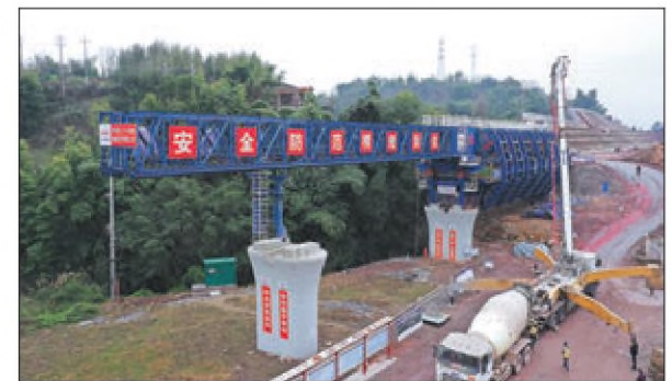
An image shows the construction site of a bridge on the Xi'an-Chongqing High-speed Railway in Chongqing last week. The railway is being built by State builders including China Railway 24th Bureau Group Corp. PROVIDED TO CHINA DAILY
