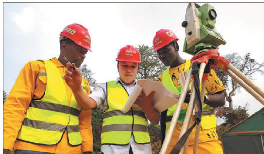
Engineers of China Railway 20th Bureau Group Corp discuss construction plans on a section of the Ntui-Mankim highway project in Cameroon last week. PROVIDED TO CHINA DAILY
