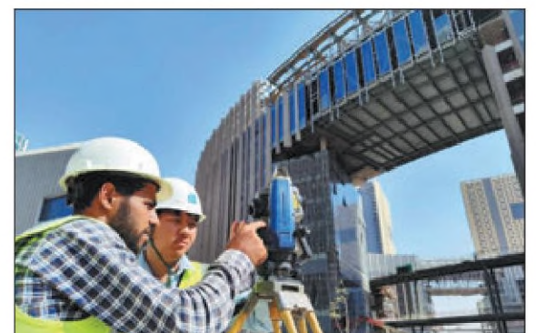
Workers from China and Egypt take measurements at the construction site of the New Administrative Capital in eastern Cairo on Sept 24. XINHUA
