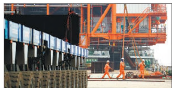
Employees work on a smart offshore oil project in Tianjin. DU PENGHUI / XINHUA
