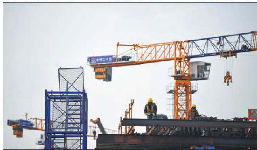
CREC employees work on a bridge project in Xi'an, Shaanxi province. ZHANG BOWEN / XINHUA
