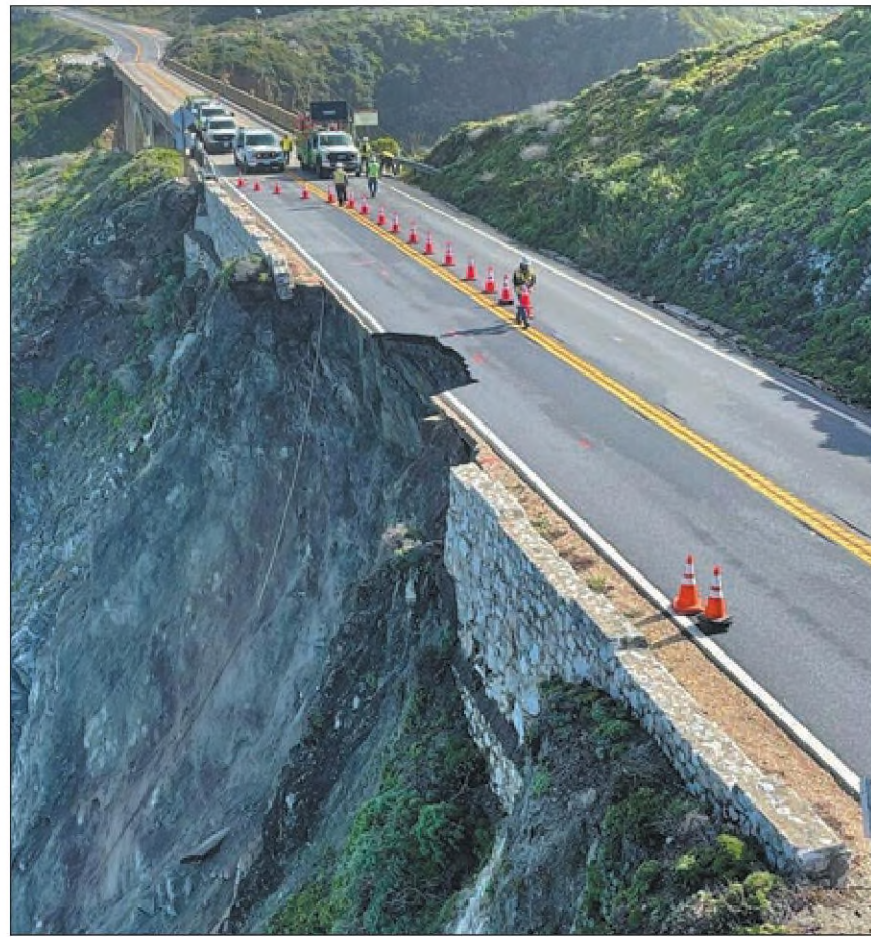
This photo shows a damaged section of Highway 1 on Sunday in the south of Rocky Creek Bridge in Big Sur, California. Authorities urged motorists to avoid the scenic highway after a section of the coastal route collapsed during an Easter weekend storm, forcing closures and stranding motorists near Big Sur, authorities said. CALTRANS' DISTRICT 5 VIA AP
