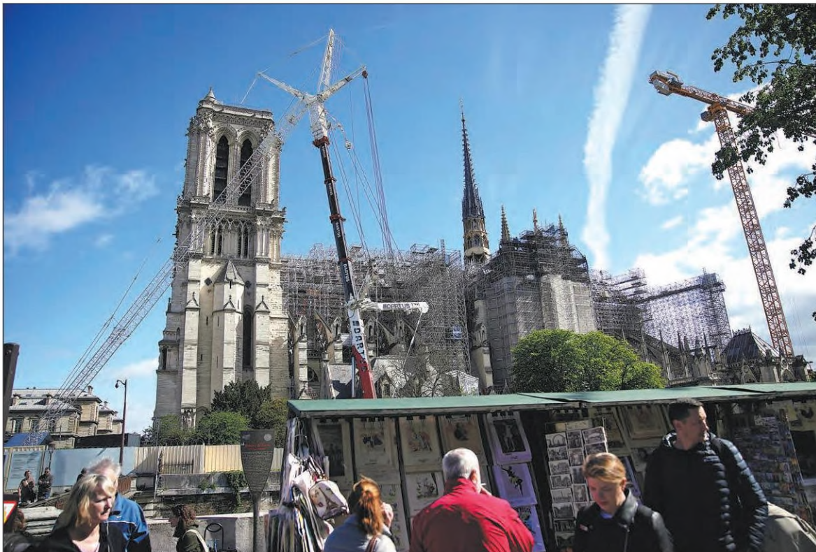
People walk past a scaffolded Notre Dame Cathedral on Monday in Paris, France. Monday marked the fifth anniversary of the devastating fire that engulfed and severely damaged the medieval structure. The process of restoring the monument is expected to be completed by the end of the year. CHRISTOPHE ENA / AP
