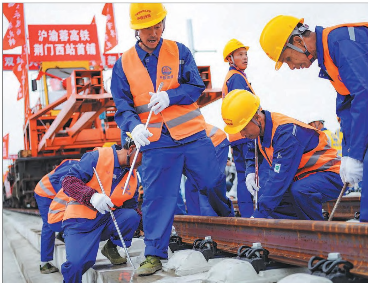
Employees of China Railway No 4 Engineering Group Co Ltd lay tracks on the Wuhan-Yichang section of the Shanghai-Chongqing-Chengdu High-speed Railway in Jingmen, Hubei province. WU HUIQIU / FOR CHINA DAILY
