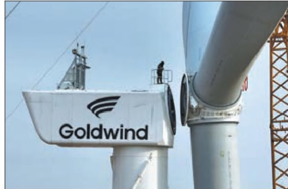
Workers install a fan blade onto a wind turbine at a power farm in Ningxia Hui autonomous region in January. YUAN HONGYAN / FOR CHINA DAILY
