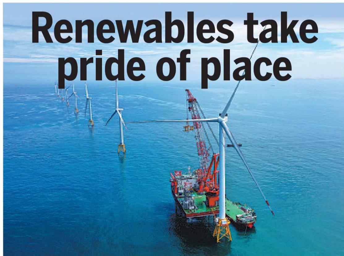
A wind turbine is assembled on an offshore platform in Fujian province in June. LIN SHANCHUAN / XINHUA
