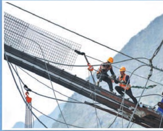
Workers install protection nets on the bridge on March 27. PHOTOS BY YANG WENBIN / XINHUA
