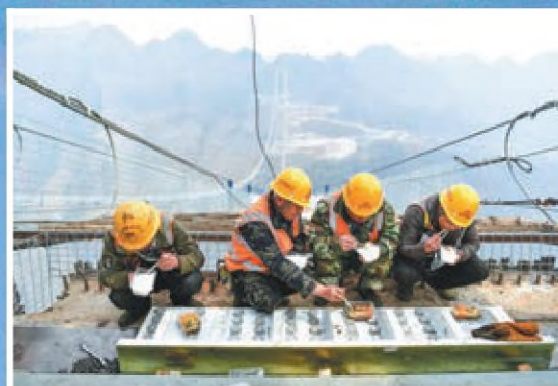
Workers eat their lunch that has been delivered by a tower crane on March 27.
