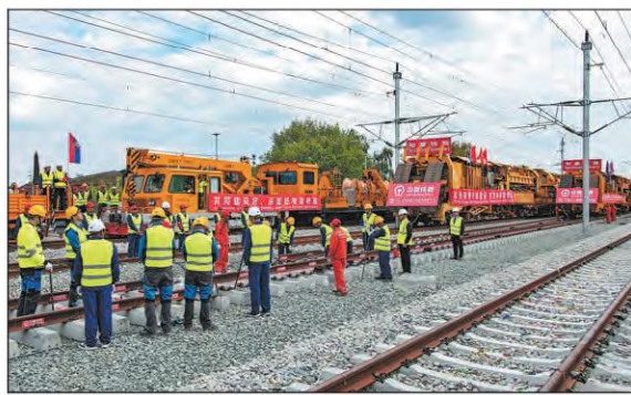
Workers lay tracks for the Novi Sad-Subotica section of the Belgrade-Budapest railway in Backa Topola, Serbia, in April. WANG WEI / XINHUA
