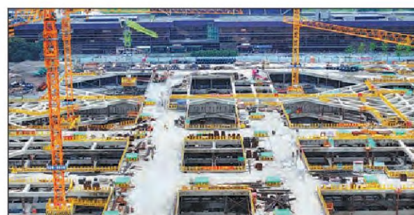
A drone image shows the construction site of the service center of Songjiang Railway Station in Shanghai. According to China Railway 24th Bureau Group Corp, a State builder participating in the project, the station will be another major transportation hub in Shanghai and link the metropolis with more major rail lines. PROVIDED TO CHINA DAILY
