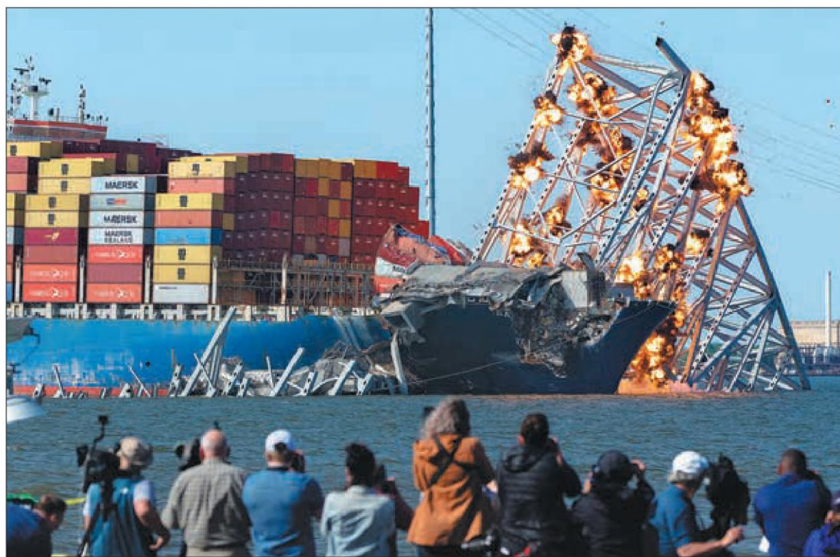
Explosives are detonated on Monday to bring down the Francis Scott Key Bridge, which partially collapsed after being hit by the container ship Dali on March 26, in Baltimore, the United States. The bridge was demolished to free the vessel that had been trapped under it for seven weeks. MARK SCHIEFELBEIN / AP
