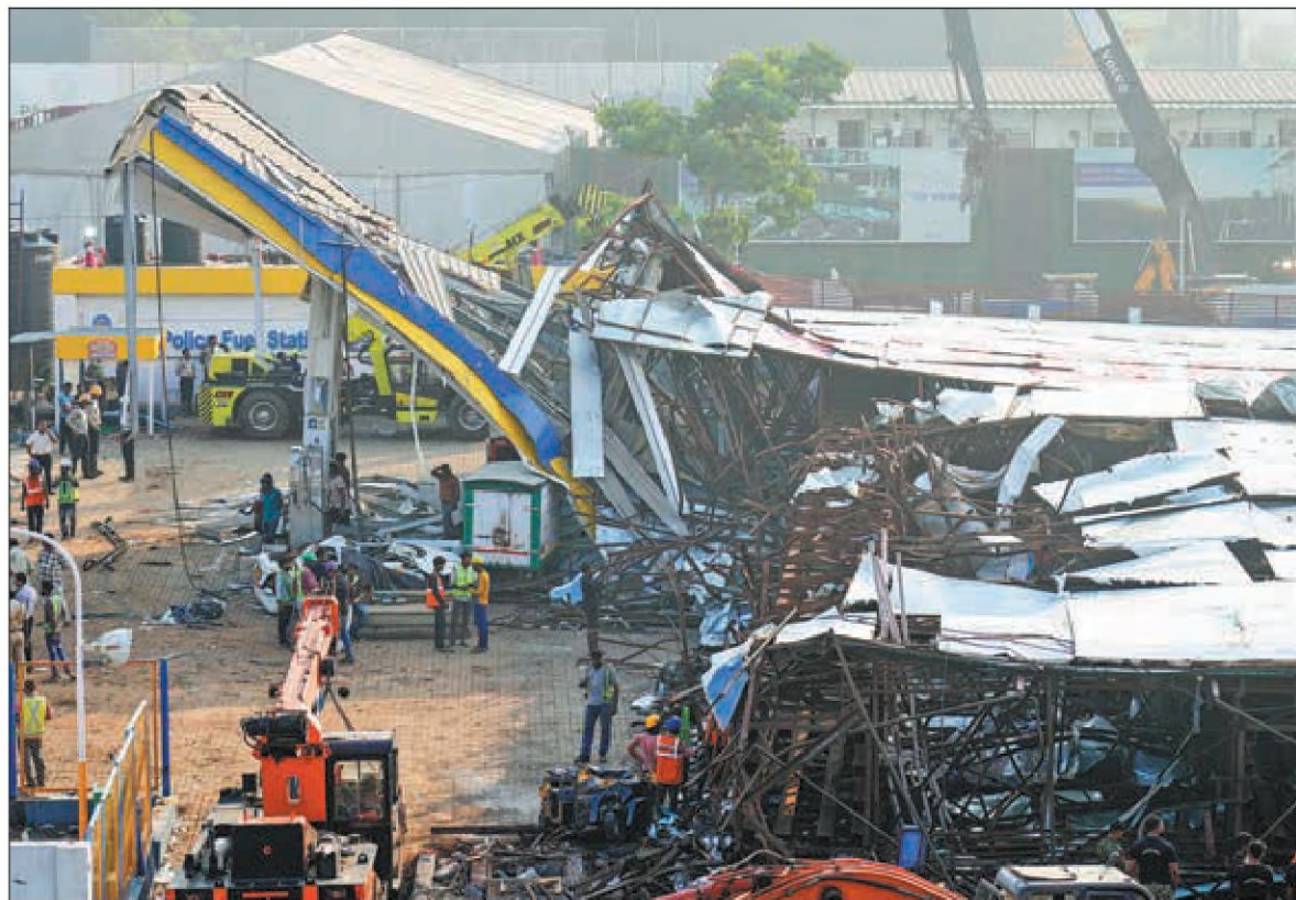
Rescuers search on Tuesday for people trapped under a huge billboard that collapsed on a fuel station on Monday evening during a severe storm in suburban Mumbai, India. Fourteen people were killed and dozens were injured in the accident. RAJANISH KAKADE / AP
