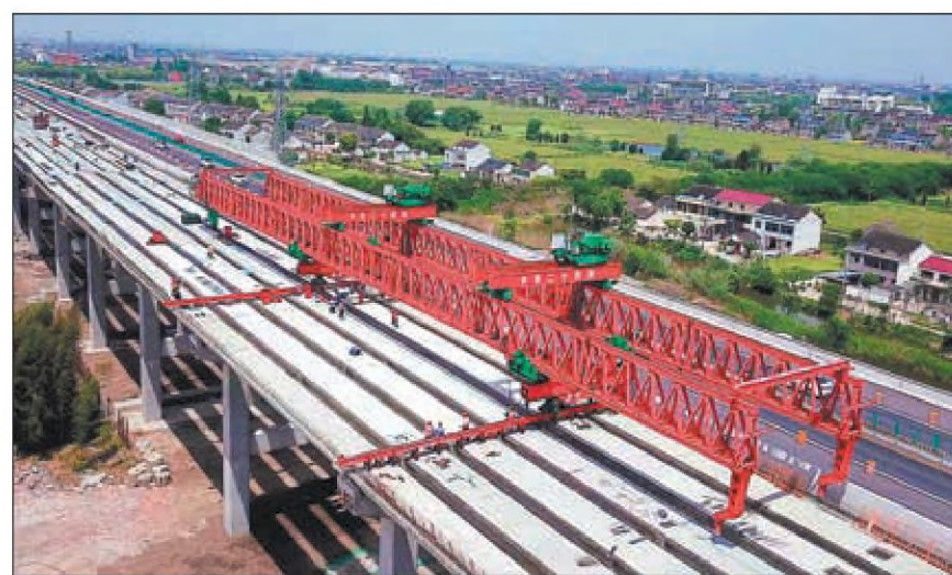
A drone image shows the construction site of a highway expansion project in Jingjiang, Jiangsu province, last week. Builders with China Railway 24th Bureau Group Corp completed installation of box girders of a major bridge, a milestone in the expansion project of the Pingchao-Guangling section of the Shanghai-Xi'an Expressway, which aims to enhance coastal-inland links. PROVIDED TO CHINA DAILY
