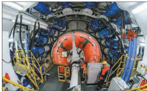
A worker conducts checks on a tunnel boring machine at a construction site for the Jintang Undersea Tunnel in Zhejiang province on Thursday. YAO FENG / FOR CHINA DAILY
