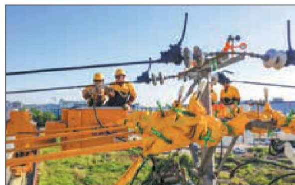
State Grid employees check transmission equipment in Huzhou, Zhejiang province. WANG ZUN / FOR CHINA DAILY
