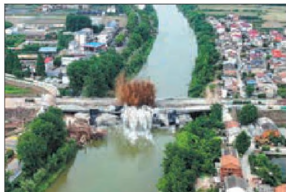
Kejiadun Bridge on the Wuhan-Huangshi Highway in Ezhou, Hubei province, which had been in service for 33 years, is demolished through controlled explosion on Sunday, giving way to the construction of a bigger bridge to accommodate increasing traffic demand. KE HAO / FOR CHINA DAILY
