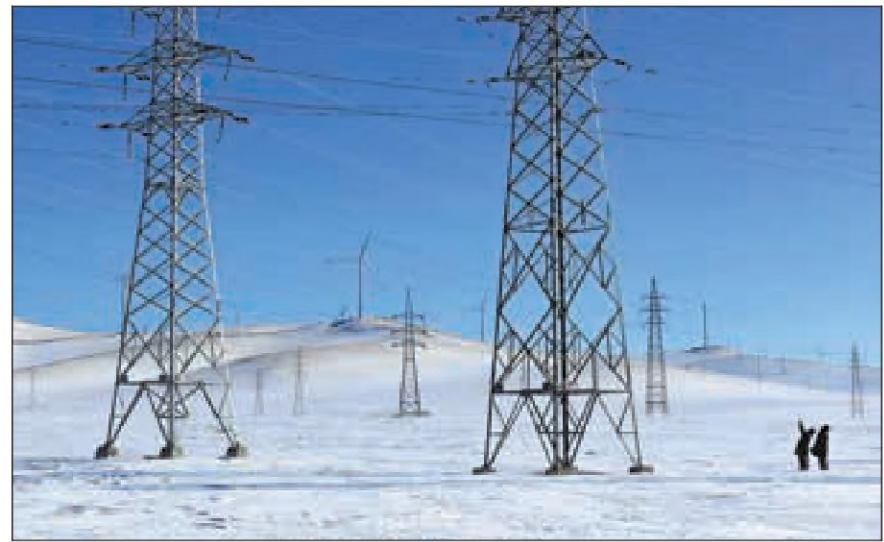
State Grid employees check power transmission lines in Tongliao, Inner Mongolia autonomous region. WANG ZHENG / FOR CHINA DAILY
