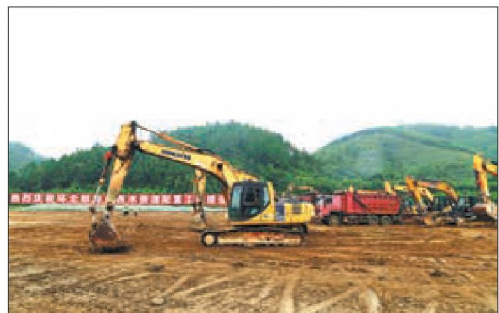
The massive water diversion project for the Beibu Gulf breaks ground in Hepu county of Beihai, Guangxi Zhuang autonomous region, in September last year. ZHOU HUA / XINHUA
