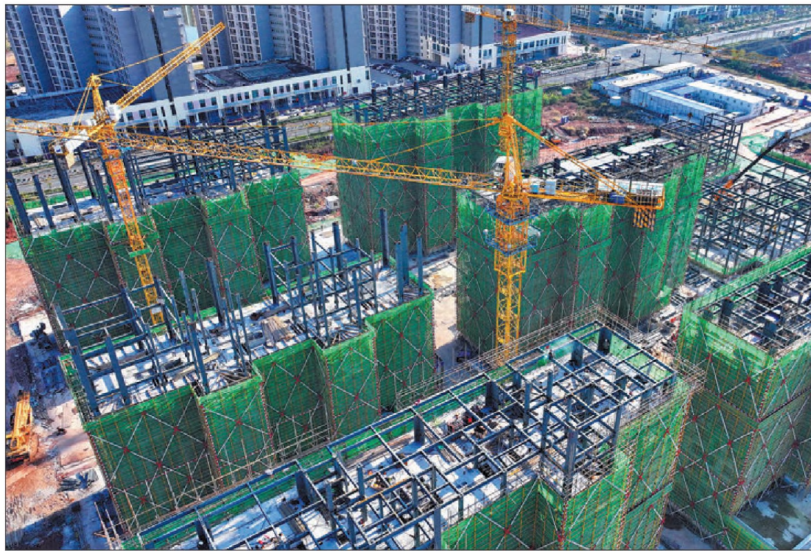
A construction site of an affordable housing project in Ganzhou, Jiangxi province, in December. ZHU HAIPENG / FOR CHINA DAILY
