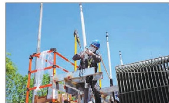
A technician from State Grid Zhejiang Electric Power Co works on a substation in Huzhou, Zhejiang province. The local branch of the State electricity supplier is helping the city by slashing the emissions of sulfur hexafluoride gases by half. It can reduce the environmental impact of equipment at the transformer station and promote carbon reductions in the local power grid. DONG ZHENMAO / FOR CHINA DAILY
