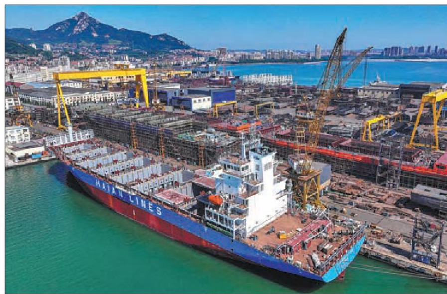
Large ships under construction at a shipyard in Rongcheng, Shandong province. LI XINJUN / FOR CHINA DAILY
