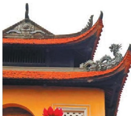
Roof decorations on Doan Mon, the southern gate of the Imperial Citadel of Thang Long in Hanoi. JIANG DONG / CHINA DAILY
