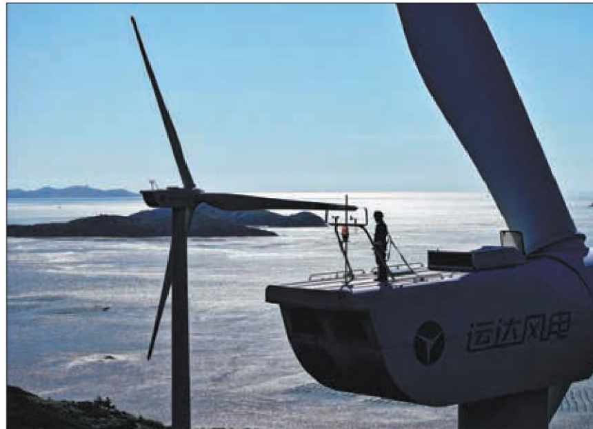
A technician conducts maintenance work at an offshore wind farm in Zhoushan, Zhejiang province, in November. YAO FENG / FOR CHINA DAILY
