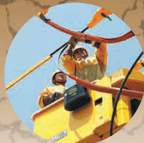
Technicians from the State Grid Yinchuan Power Supply Company work in the heat in Yinchuan, Ningxia Hui autonomous region, on Friday.
