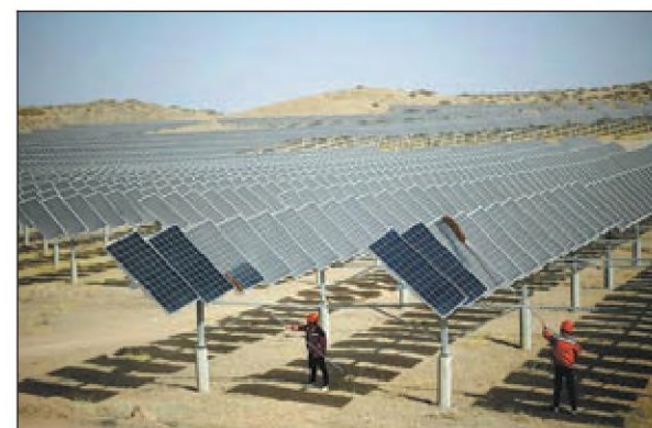
Workers dust photovoltaic panels after windy weather at a power station in Yinchuan, Ningxia Hui autonomous region, in March 2023. WANG PENG / XINHUA
