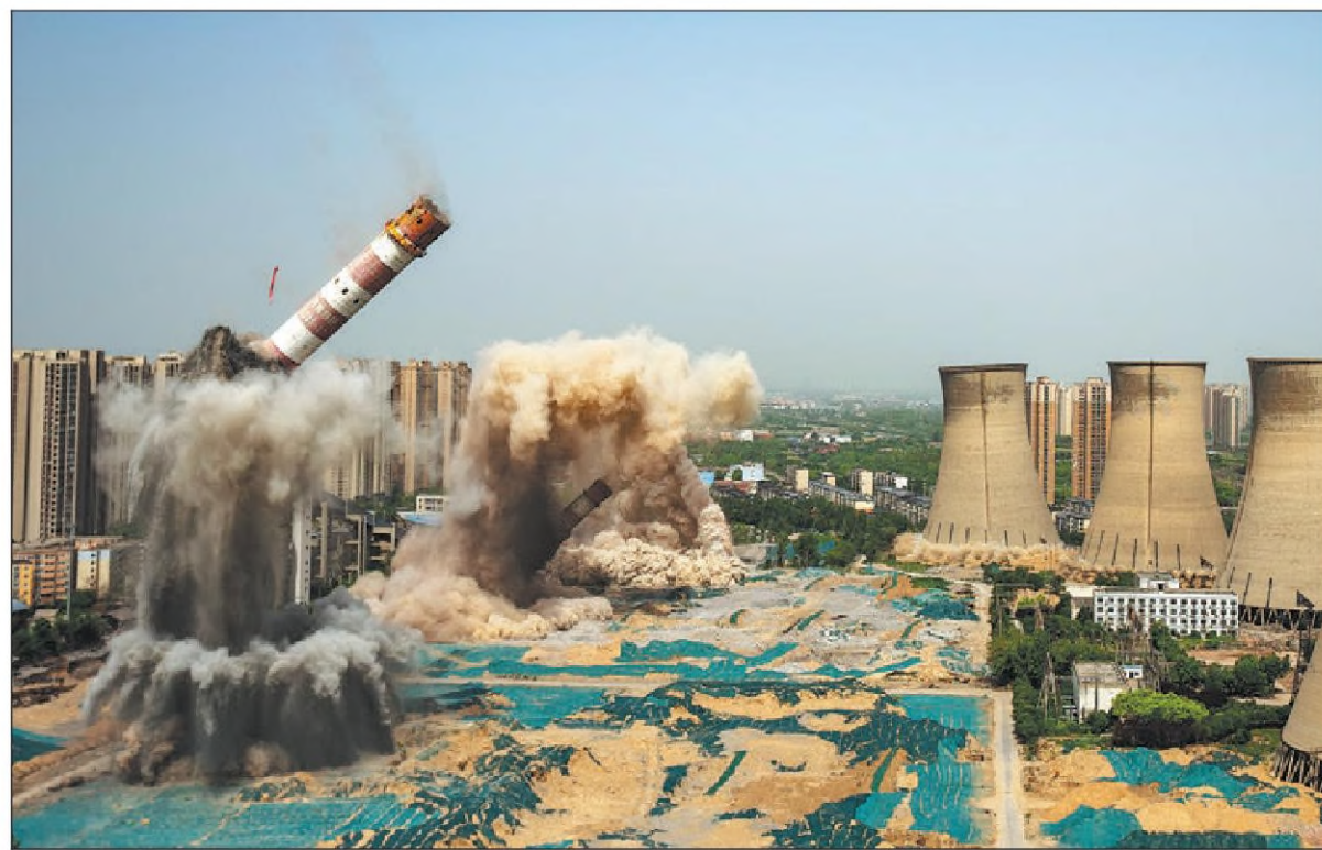
Chimneys collapse in clouds of dust after being detonated in Zhengzhou, Henan province, on Tuesday. In about 20 seconds, three 210-meter chimneys and three of the five 105-meter cooling towers that were part of a thermal power station were demolished. The plant, now surrounded by residential buildings and greenery, shut down in 2019. The two remaining cooling towers will serve as industrial scenery when the land is repurposed. BAI ZHOUFENG / FOR CHINA DAILY
