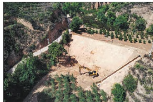
An excavator works on enhancing a warp-land dam in Xindiangu in Suide, Shaanxi province, on Sunday. The dam helps intercept eroded soil and boost agricultural production. LI HE / XINHUA
