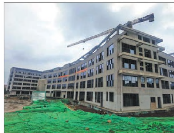
An image shows the construction site of a hospital in Kunming, Yunnan province. Construction of the hospital has been undertaken by China Railway 23rd Bureau Group Corp as a key local livelihood project as it is the first comprehensive hospital in the Kunming Airport Economic Zone. The project is close to completion and is undergoing interior decor work. PROVIDED TO CHINA DAILY
