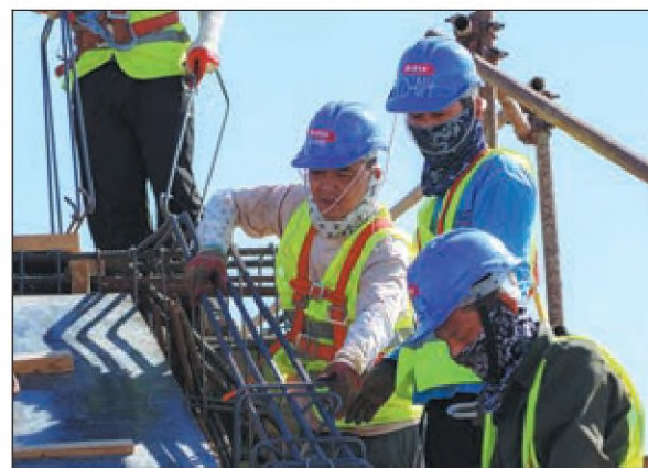
Chinese builders work at the construction site of the Olympic City project in Tashkent on Aug 13 last year. XINHUA
