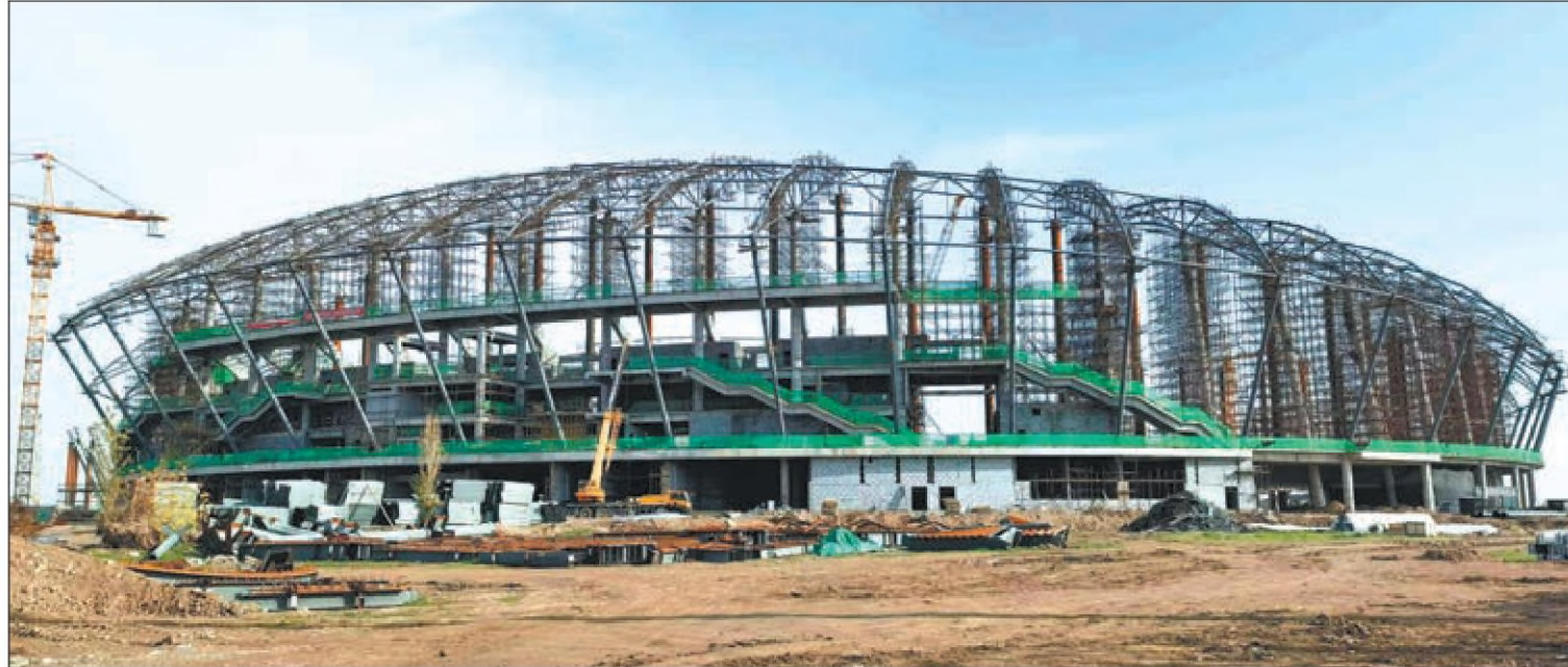
The Olympic City is under construction by China CAMC Engineering Co in Tashkent, Uzbekistan, a member of the Shanghai Cooperation Organization, on Jan 1. XINHUA
