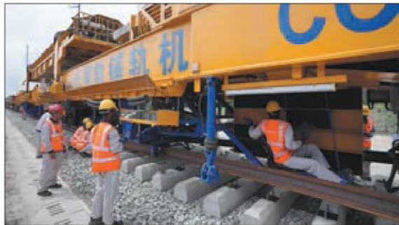
Workers lay down the first track for the East Coast Rail Link project in Gebeng, Pahang state, Malaysia, on Dec 11. VINCENT THIAN / AP
