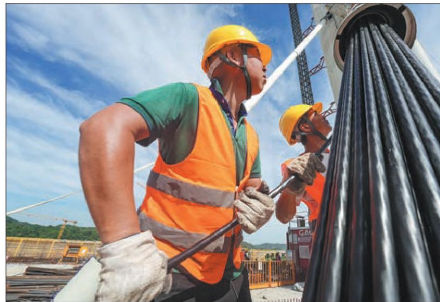
CREC4 employees install steel strands at a swivel cable-stayed bridge traversing Lushan Railway Station in Jiujiang, Jiangxi province. SHEN JIAPENG / FOR CHINA DAILY
