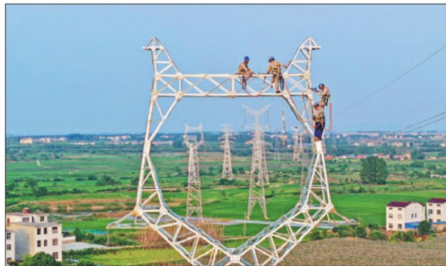
Technicians check a power transmission tower in Chuzhou, Anhui province. SONG WEIXING / FOR CHINA DAILY
