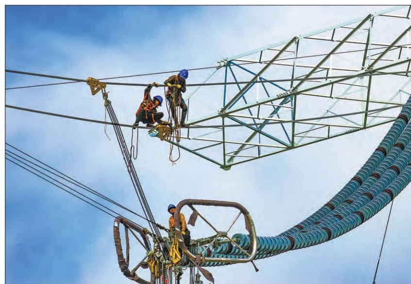
Employees check a power transmission network in Zhangye, Gansu province.
