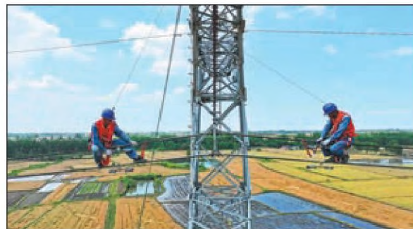
Top: A power staff member (right) offers electricity usage guidance to a farmer in Yinchuan, Ningxia Hui autonomous region, in June. YUAN HONGYAN / FOR CHINA DAILY Above: Employees carry out maintenance work on transmission lines in Chuzhou, Anhui province, in May. SONG WEIXING / FOR CHINA DAILY
