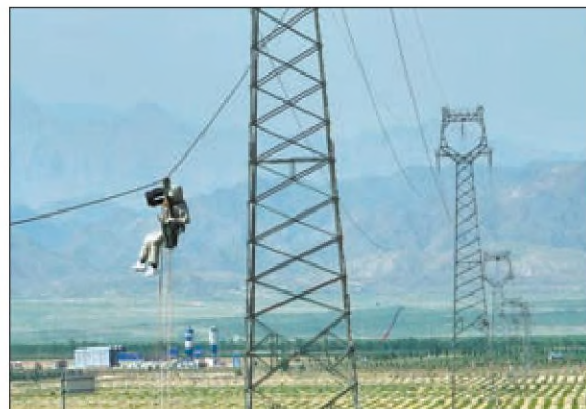
A technician inspects power transmission cables by using "flying man" equipment in Yinchuan, Ningxia Hui autonomous region, in June. YUAN HONGYAN / FOR CHINA DAILY
