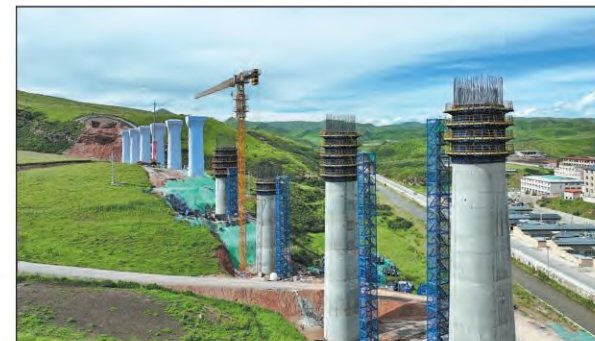
Piers of a railway bridge leading to the 8.35-kilometer Liren Tunnel are seen under construction in Gansu province on Thursday. Built by China Railway No 4 Engineering Group Co Ltd, the bridge and the tunnel are part of the Sichuan-Qinghai Railway, which aims to cut travel time between the two inland provinces. XING JIANG / FOR CHINA DAILY
