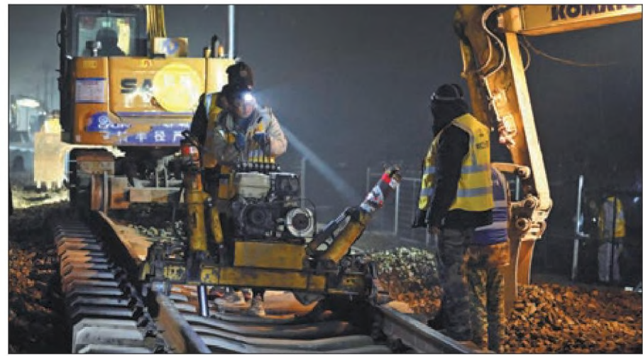
Construction employees of China Railway 24th Bureau Group Corp lay tracks at the new Hefei West Railway Station in Anhui province. The State builder said on Friday it has completed relocating the lines of the Hefei-Fuzhou High-speed Railway, a move to expand the railway station, facilitating Hefei's efforts to build itself as a transportation hub in East China. ZHOU MU / XINHUA
