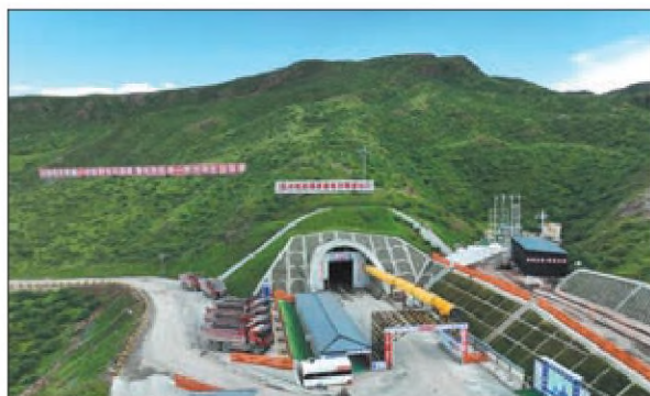
Builders from China Railway No 4 Engineering Group Co Ltd work in Gansu province on Tuesday on the exit for the Gol Tunnel on the Gansu-Qinghai section of the Sichuan-Qinghai Railway which links the capitals of Sichuan and Qinghai provinces. The railway is expected to be completed within six years. XING JIANG / FOR CHINA DAILY
