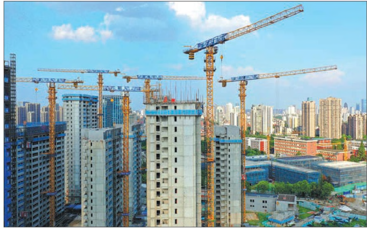
A residential property project is under construction in Hefei, Anhui province. CHEN SANHU / FOR CHINA DAILY
