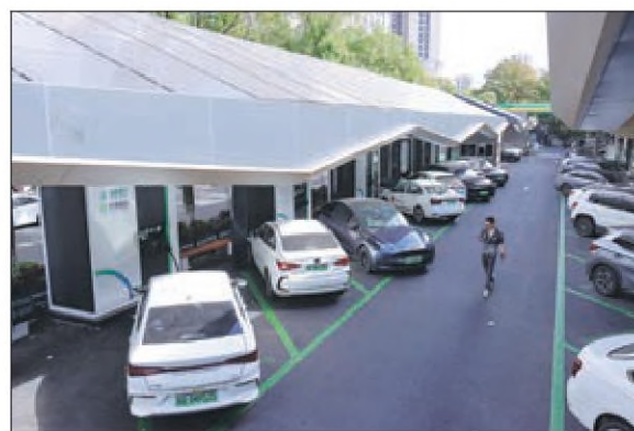
Charging piles seen on a street in Changzhou, Jiangsu province. WANG QIMING / FOR CHINA DAILY
