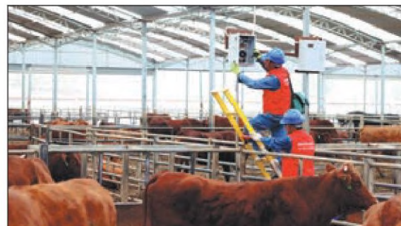
Employees of State Grid Ningxia Electric Power Co check power equipment at the Yanghe Cattle Raising Base in Longde county in the Ningxia Hui autonomous region, which is part of the SOE's efforts to support the local cattle business. LIU HUI / FOR CHINA DAILY
