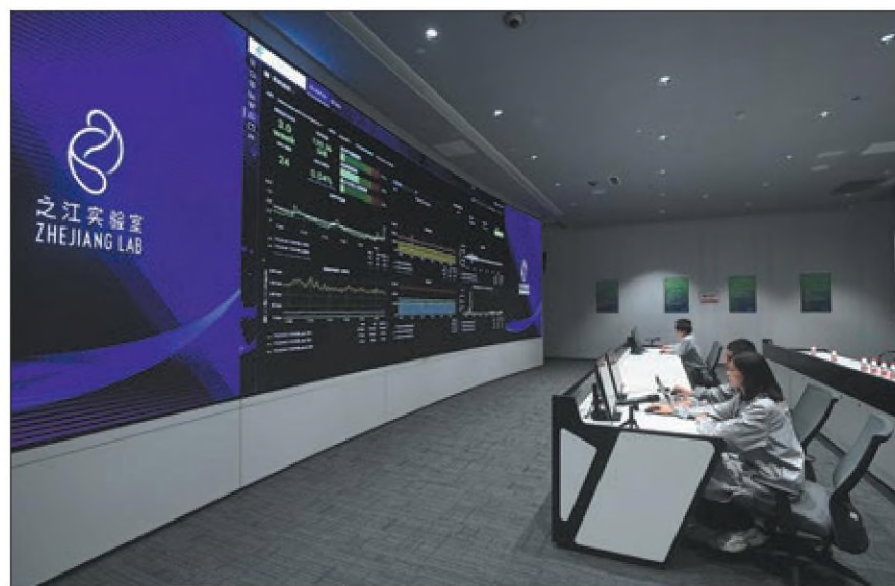
Top: A robot (left) inspects operations at a net-zero emissions data center in Haidong, Qinghai province, in March. LI JUN / CHINA NEWS SERVICE Above: Technicians track server status at Zhejiang Lab in Hangzhou, Zhejiang province, in June 2022. HUANG ZONGZHI / XINHUA
