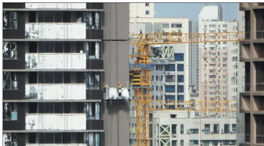
A construction crew works at a housing project in Shanghai in June. WANG GANG / FOR CHINA DAILY
