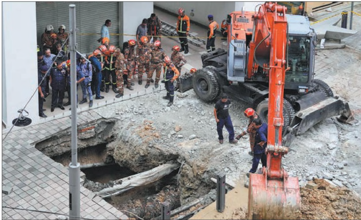
Fire and rescue departments use crane to dig after receiving reports that a woman has fallen into the sinkhole after a section of the sidewalk caved in Kuala Lumpur, Malaysia, on Aug 23. VINCENT THIAN / AP
