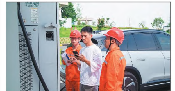
Employees of State Grid Quzhou Electric Power Co help a motorist charge his electric vehicle at a service area along the G60 Shanghai-Kunming Expressway. The power operator of Quzhou, Zhejiang province is ramping up inspections to ensure safe electricity use during the upcoming Mid-Autumn Festival and National Day holidays. MAO XIAOWEI / FOR CHINA DAILY
