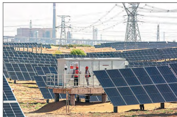
Technicians carry out inspections at a solar power farm in Hanggin Banner, Inner Mongolia autonomous region, in June. MEI TAO / FOR CHINA DAILY
